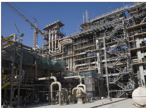
Construction is nearly complete on the 7.8-million-tons-per-year RasGas liquefied natural gas (LNG) Trains 6 and 7 in Qatar.
