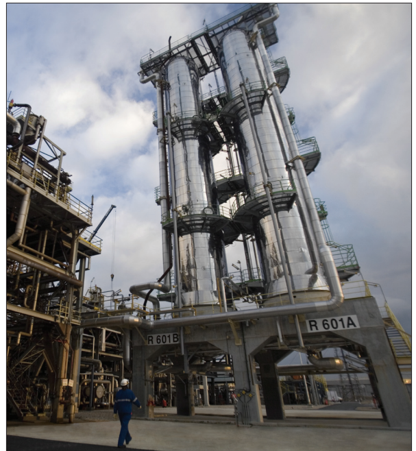
New facilities to reduce diesel sulfur were installed at our Port-Jerome-Gravenchon refinery in France.
